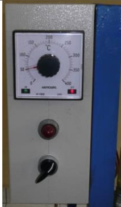
Gambar 6. 10 Panel distilator temperature control
