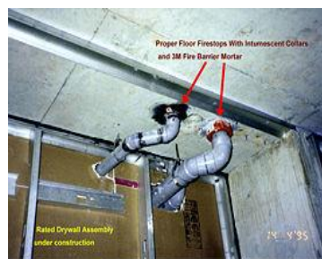
Northtown Castles, North York (now Toronto), Ontario, Canada, April 1995: Set-up for subsequent code infraction in plastic pipe wall penetrations: improper hole sizing. Firestops (in the walls) the plumber considered to be the drywall's responsibility. If floor openings are properly done in this case, with intumescent pipe collars and firestop mortar. The intumescent will expand and choke off the melting pipes. Drywall mud does not work as a plastic pipe firestop in the wall.
