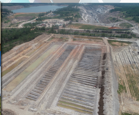
Large-scale swampy forest technology development for acid mine drainage management in 53 ha of void
