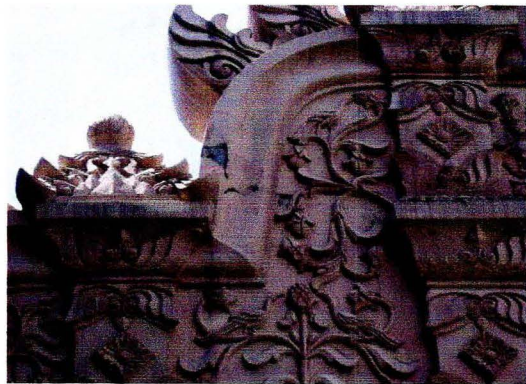
The damage on the south outer wing's corner
