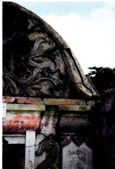
Crack on the south side of urung-urung entrance gate's roof
