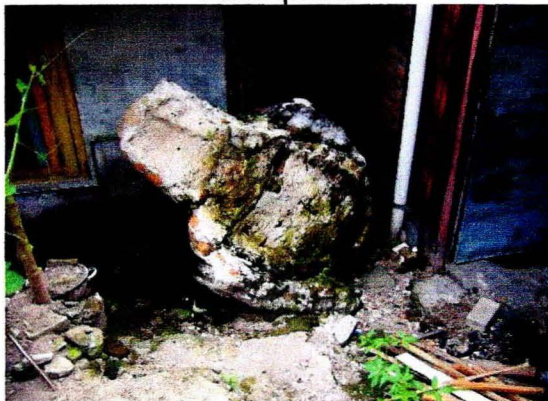
The collapsed pekxi beri in detail
