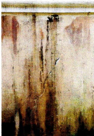
Cracks on the west inner fence structure of the Gedong Sekawan
