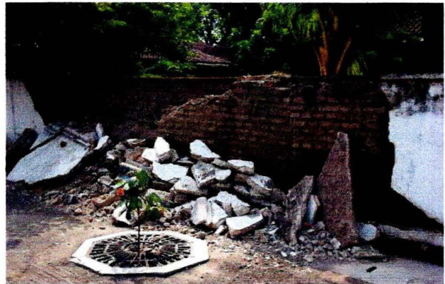
The condition of the wall on the north of Saka Tunggal mosque
