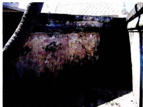
Cracks on the west outer fence structure of the Gedong Sekawan
