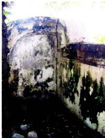
Cracks on the north outer fence structure of the Gedong Sekawan
