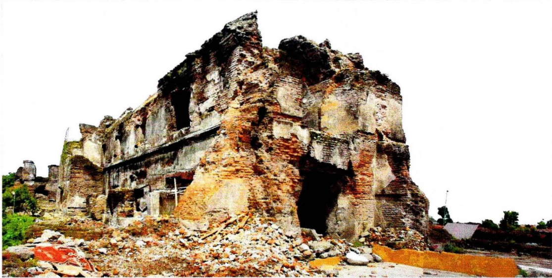
The condition of Pulo Kenanga from northeast view
