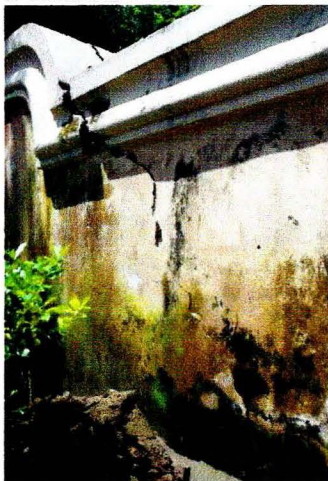
Cracks on the south inner fence structure of the Gedong Sekawan
